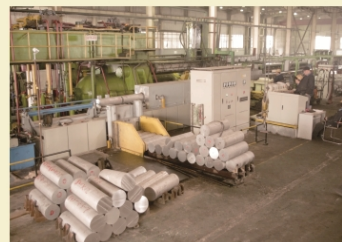
254mm铝棒变频梯度加热炉用于天津银禧铝业 254mm Aluminum Bar Frequency Conversion Induction Gradient Heating Furnace
