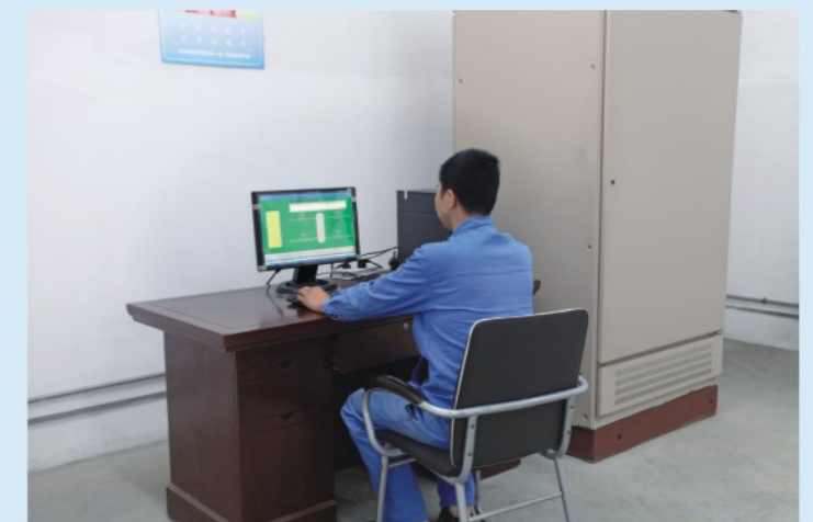
电泳涂料生产自动化PLC电脑控制系统 PLC computer control system for automated production of electrophoretic paint
