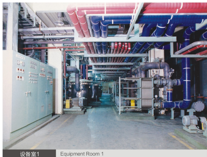
设备室1 Equipment Room 1
