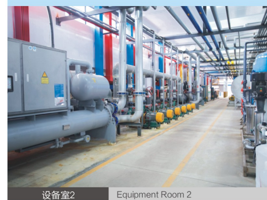
设备室2 Equipment Room 2
