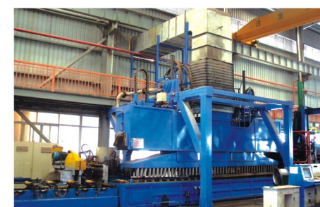
在线淬火、风水冷却设备 Online quenching, air cooling equipment
