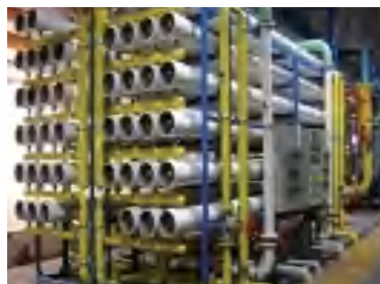
RO装置 Reverse osmosis device
